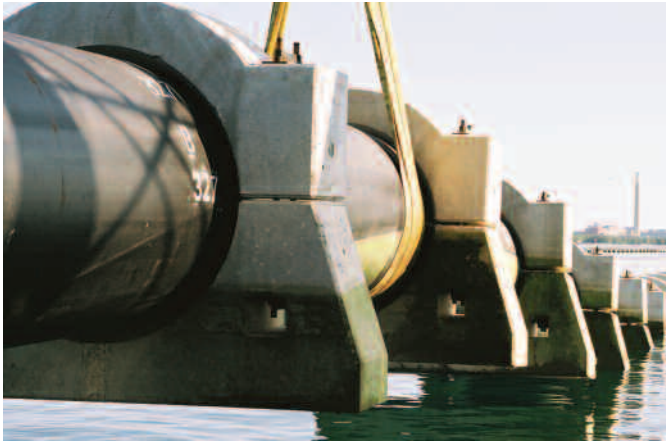
Toronto's Deep Lake Water Cooling project uses the cooling ability of the icy cold lake water for air conditioning downtown buildings (Enwave Energy Corporation)
