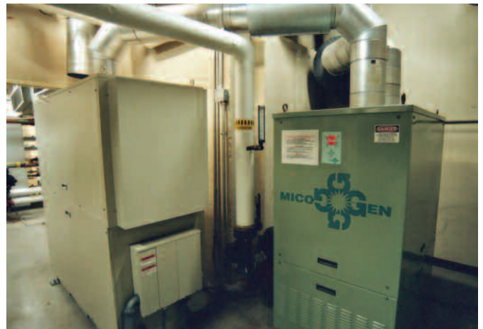
CHP at a bank. The use of CHP is especially advantageous for sites with large heating loads (Capstonen Turbines)
