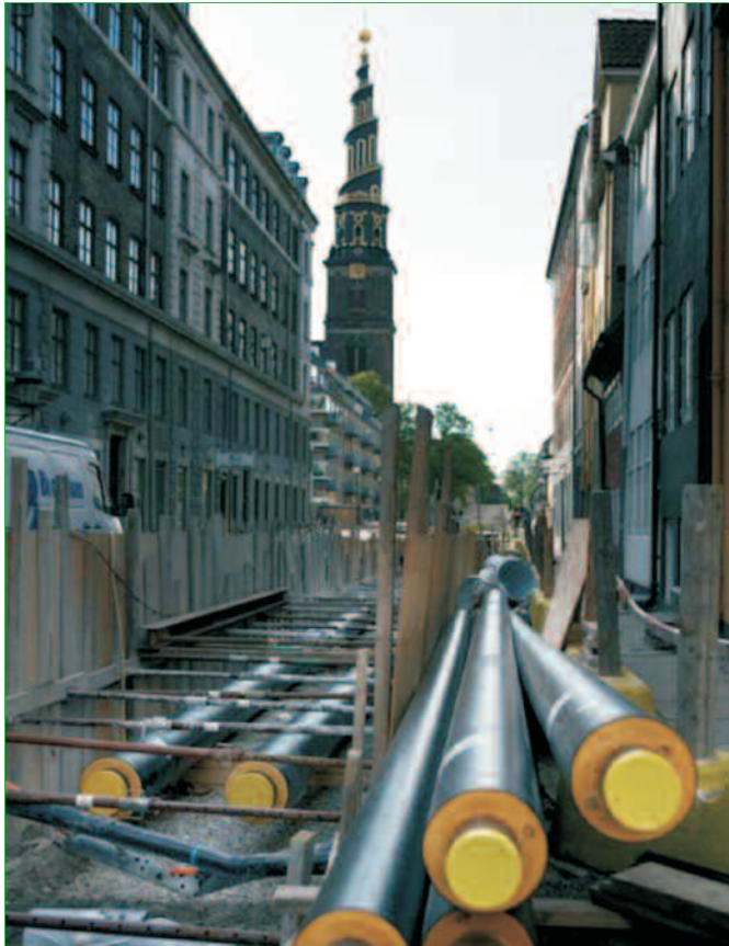
District heating pipes being installed. When combined with cogeneration, DH offers significant energy saving (Løgstør Rør)
